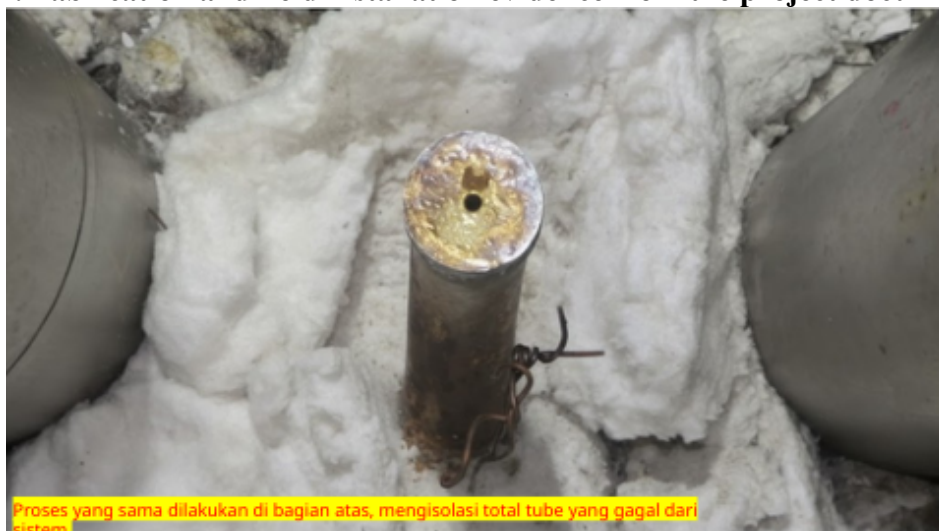
Figure 5. Example of the upper-side plugging condition after isolation of the failed tube.
